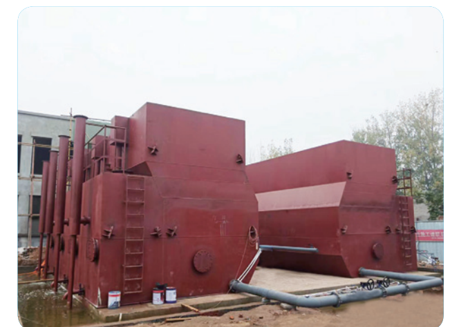
Henan Xuchang River Water Purification Project
