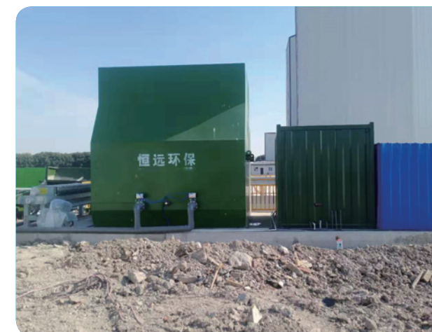
Shanxi Taiyuan 3200 square meters water purification project
