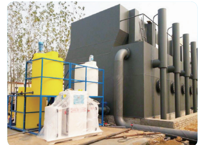
Jiangsu Nantong 5500 square meters water purification project
