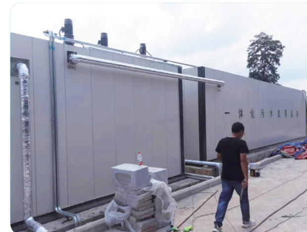
Shaanxi Baoji Expressway Service Area Sewage Treatment Project
