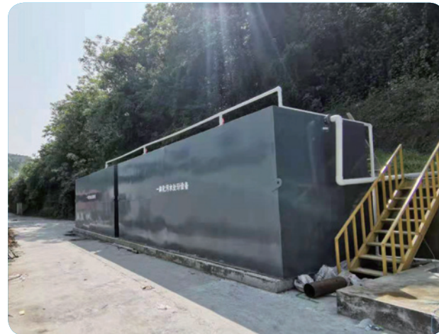
Hubei Yichang Slaughterhouse Wastewater Project
