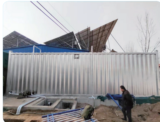
Jiangxi Jiujiang Enterprise Sewage Treatment Project
