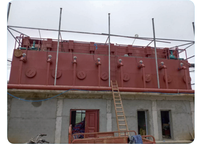
Hubei Huangshi 4800 square meters water purification project
