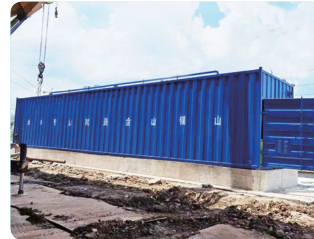
Wuhan, Hubei 500 tons/day sewage treatment project
