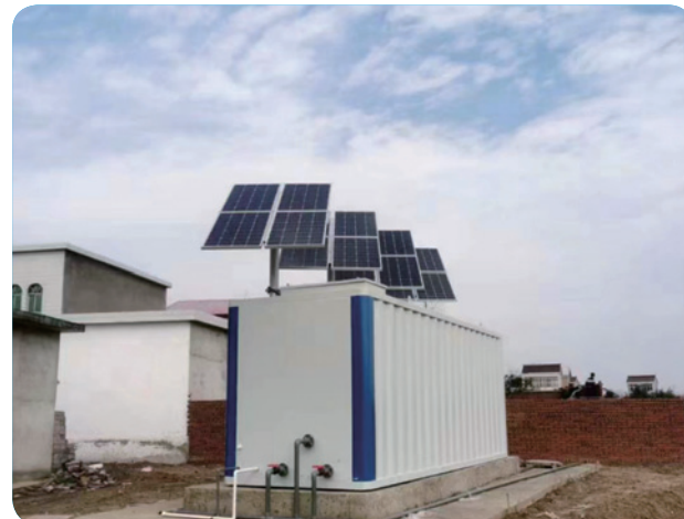
Anhui Hefei New Rural Solar Sewage Treatment Project
