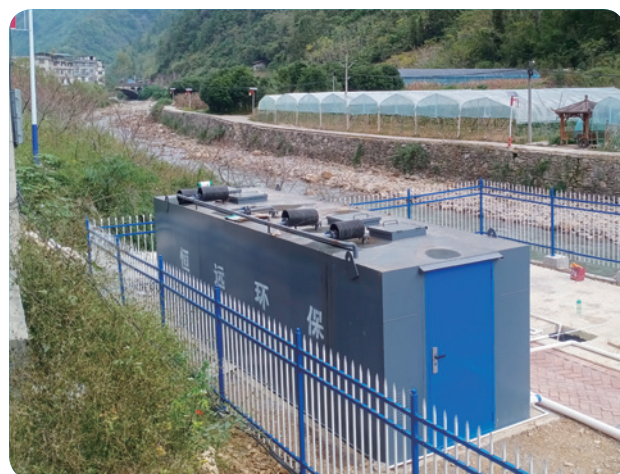
Hubei Enshi New Rural Sewage Treatment Project
