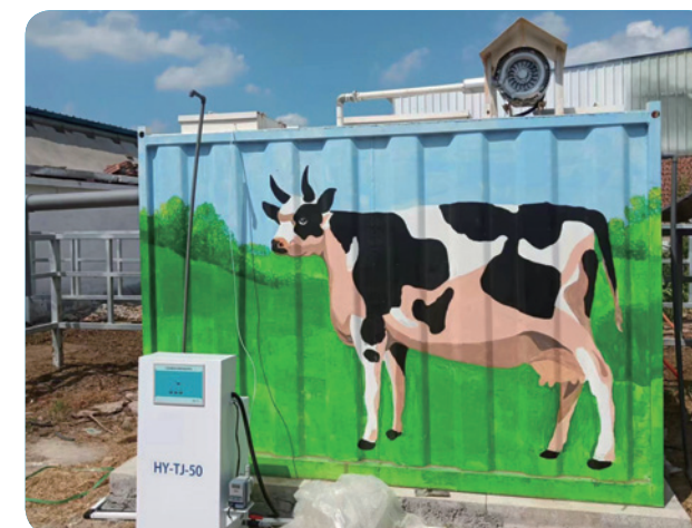
Shandong Zibo cattle farm sewage treatment project
