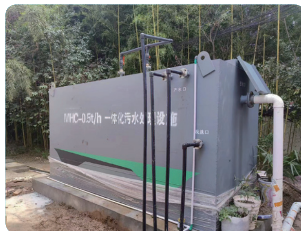
Shaanxi oil depot domestic wastewater treatment project
