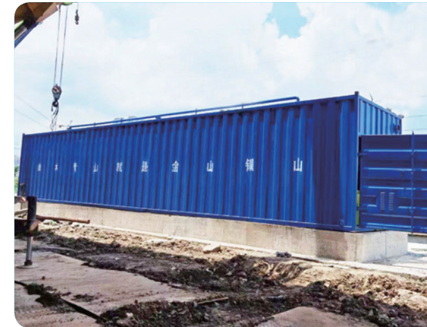
Wuhan, Hubei 500 tons/day sewage treatment project
