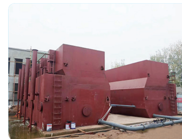
Henan Xuchang River Water Purification Project
