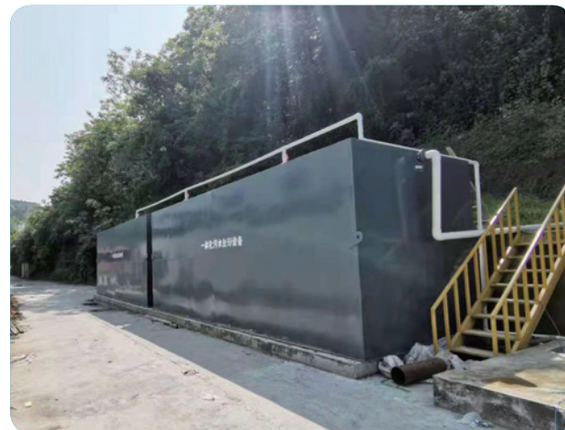
Hubei Yichang Slaughterhouse Wastewater Project
