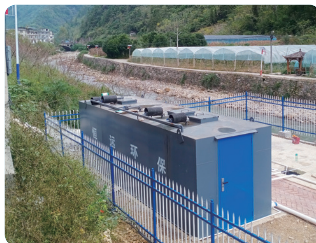
Hubei Enshi New Rural Sewage Treatment Project
