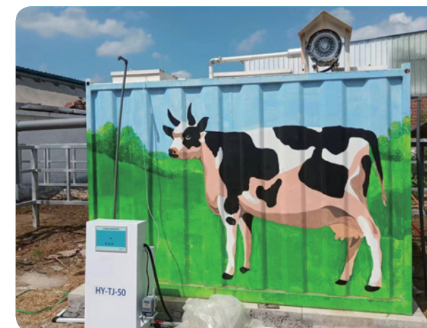
Shandong Zibo cattle farm sewage treatment project
