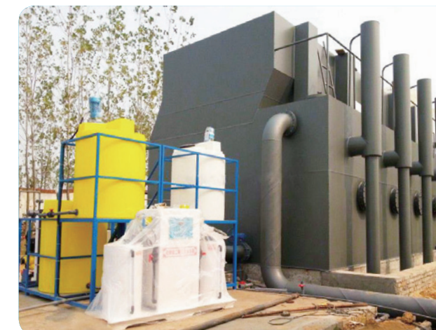
Jiangsu Nantong 5500 square meters water purification project
