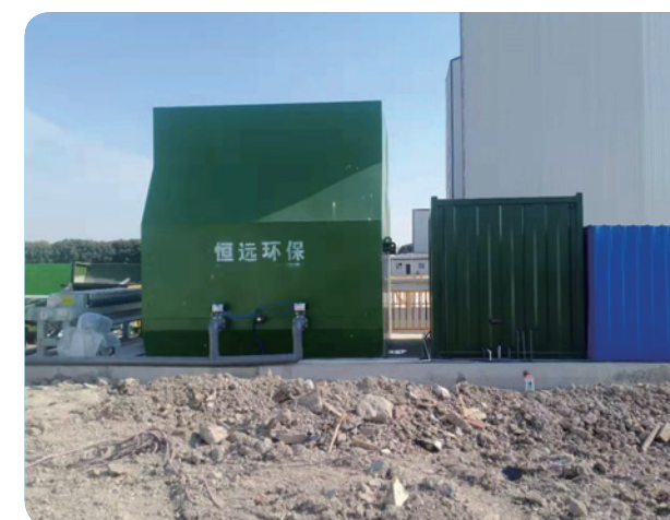
Shanxi Taiyuan 3200 square meters water purification project
