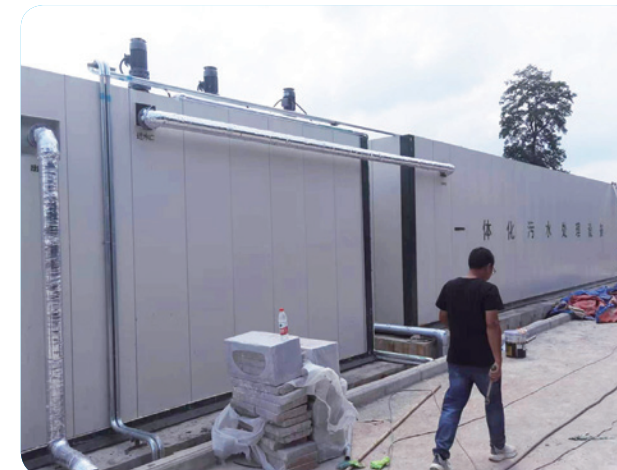
Shaanxi Baoji Expressway Service Area Sewage Treatment Project
