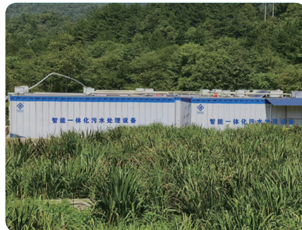
Anhui Yuexi Sewage Treatment Plant Project
