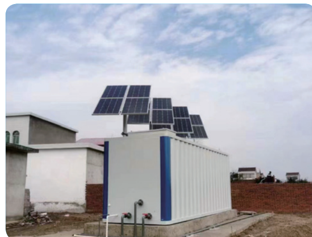
Anhui Hefei New Rural Solar Sewage Treatment Project
