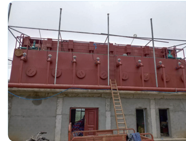
Hubei Huangshi 4800 square meters water purification project
